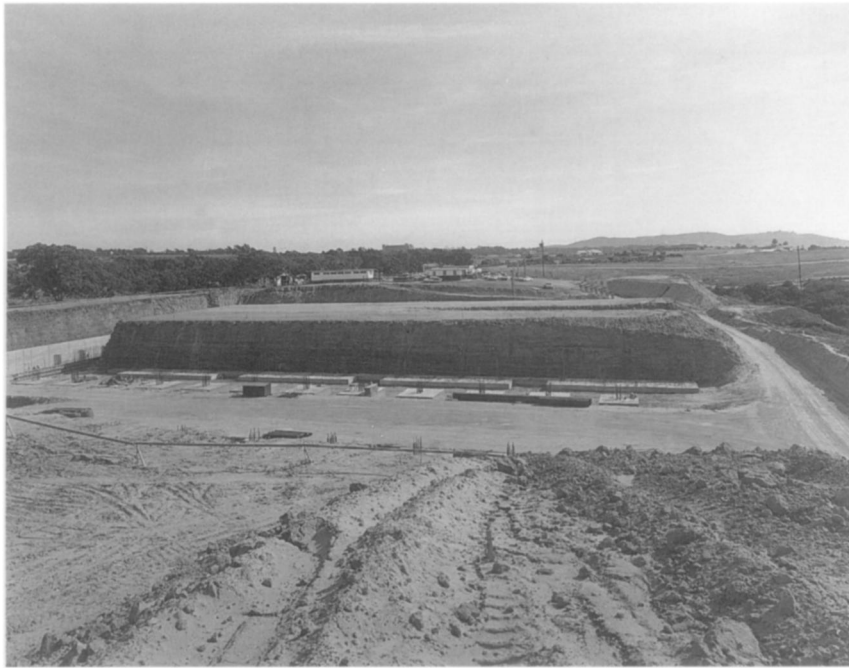
Figure 3 Construction of the Salk Institute's laboratory blocks required moving considerable amounts of earth, leaving a flat-topped mound, which become the courtyard
